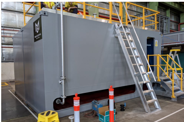
Figure 5-Mini module with a pump & pipe skid (Photo)
